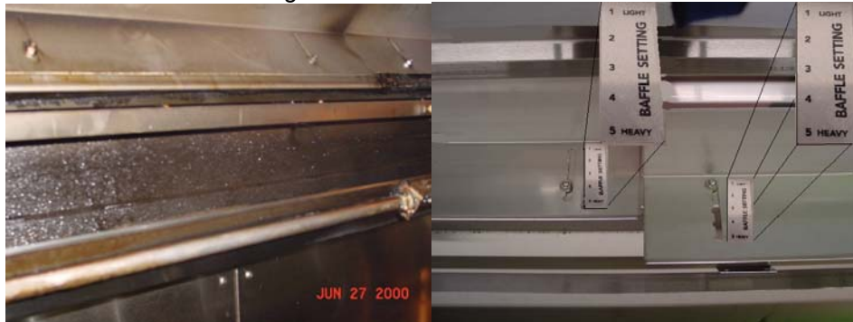
Inspect Baffle Positions
